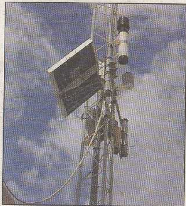
PHOTO BY VIVIAN MCMAHON This space-age-looking contraption at Big Carlos Pass can fool lightning, transmit radio signals, and measure rainfall, humidity, temperature and barometric pressure.
